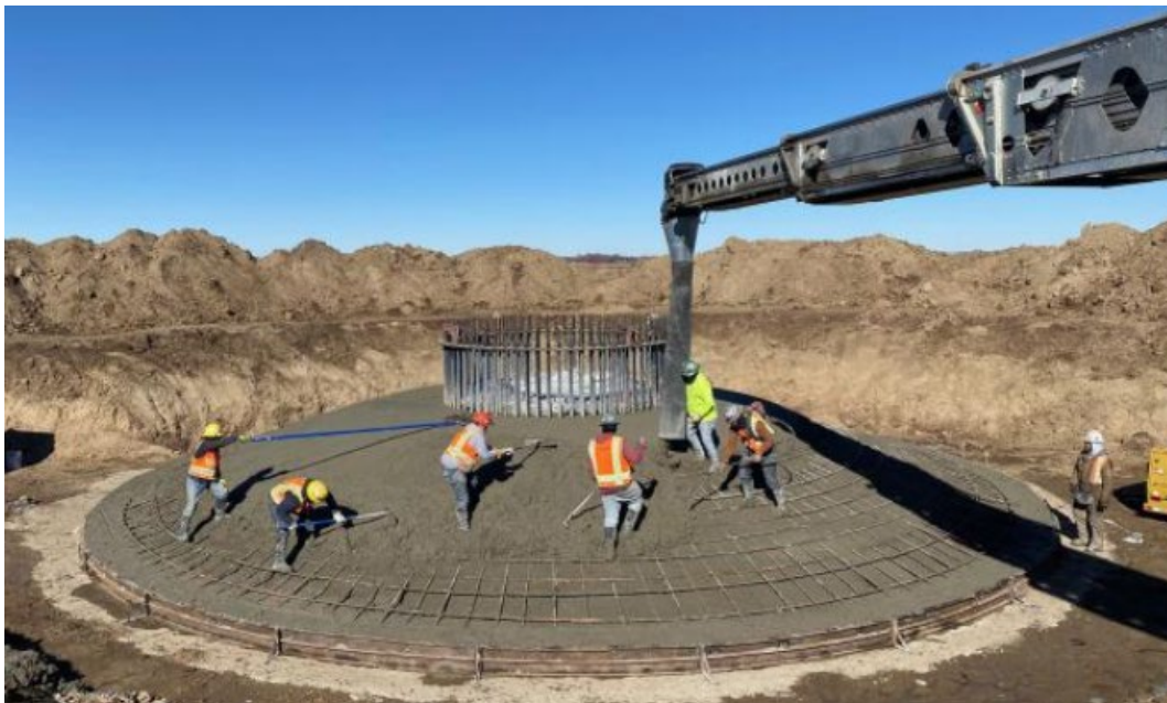
Foundation of a wind turbine can be more than 20 m in diameter and planted 3 m deep. Image from: https://www.backroadsnews.com/news/wind-turbine-construction-expected-begin-next-week
